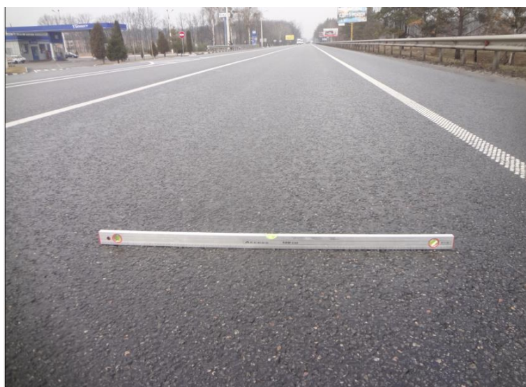
Figure 9 – Lack of rutting on a straight section
